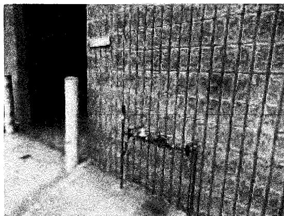
RPBP 51, outside Trash Room Bldg D along wall on sidewalk
