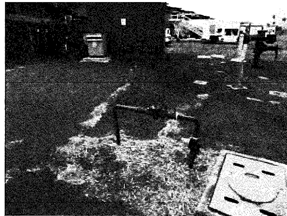
RPBP 54, on asphalt paved area next to underground meter vault, near bollards
