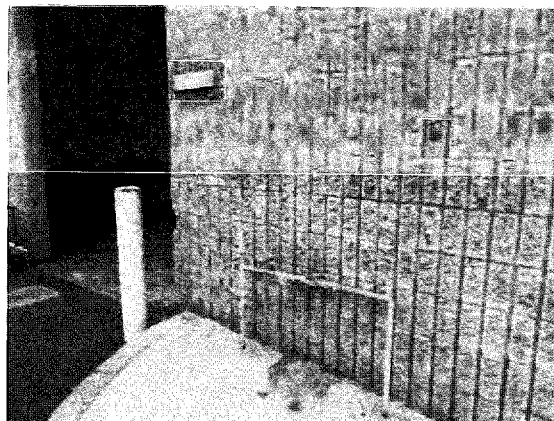
RPBP 50, outside Trash Room Bldg C along wall on sidewalk
