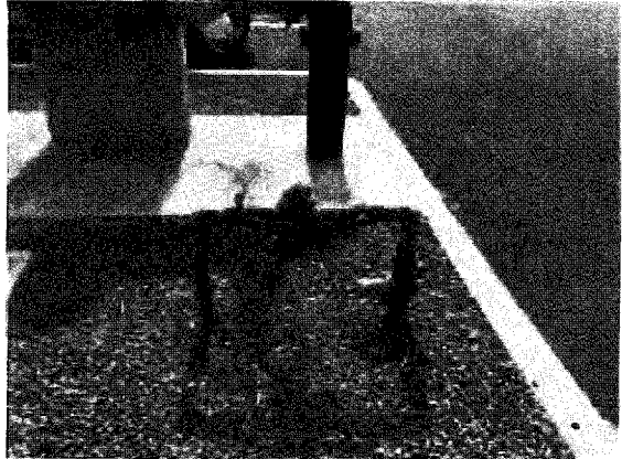
RPBP 08, In gravel area of open parking, adjacent to 8" RPBP #07
