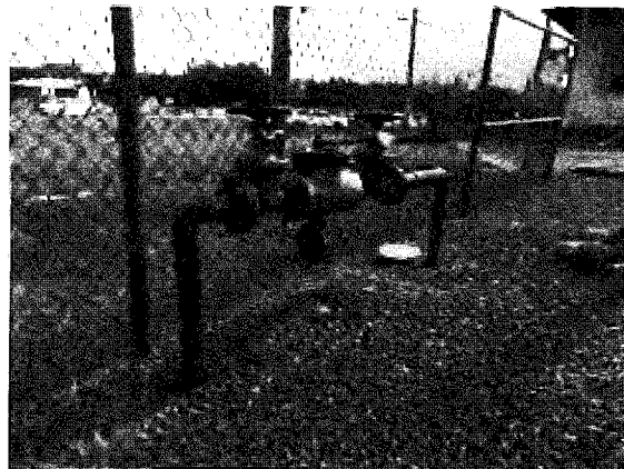
RPBP 16, Inside fenced area, north side of baseyard, right of entry gate
