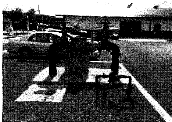
RPBP 07, in gravel area of open parking, adjacent to 2" RPBP #08
